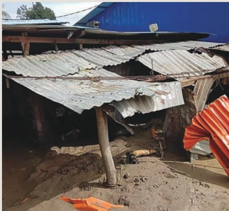
Mud damaged house
