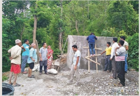
The water tank outlet in the community, connected to the solar powered irrigation pump
